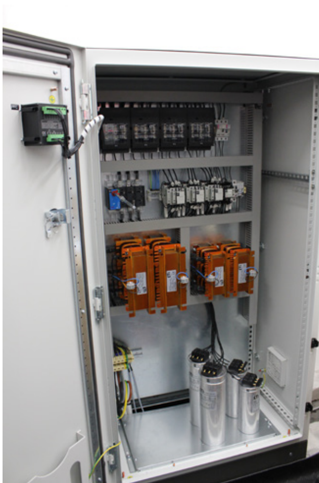
Automatic Power Factor Correction Banks
